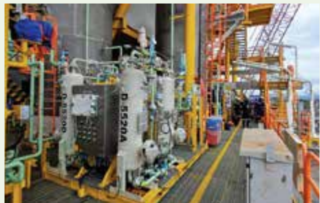
Air Compressor & Air Dryer package of VLAP at F^ Offshore Platform by Exact Automation
